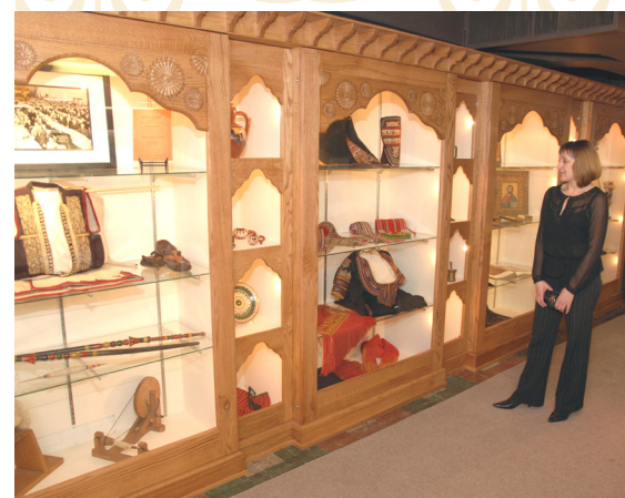
Phase One renovations included the installation of new cabinets in the former dungeon area and in the museum. Pictured is Smilena Atanassova. (Photo: Kamen Bonev)
